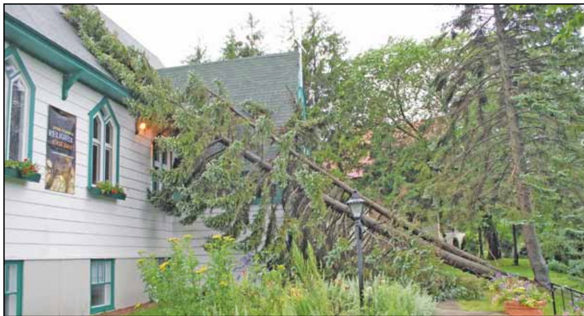
TIMBER! – The remnants of tropical storm Irene blew two large tree limbs onto the Church of St. Andrew and St. George in Baie-Comeau on Aug. 28. Damage to the church building was minimal. The storm whipped up winds as strong as 95 km/h and knocked out power to nearly 250,000 homes in eastern Quebec.
